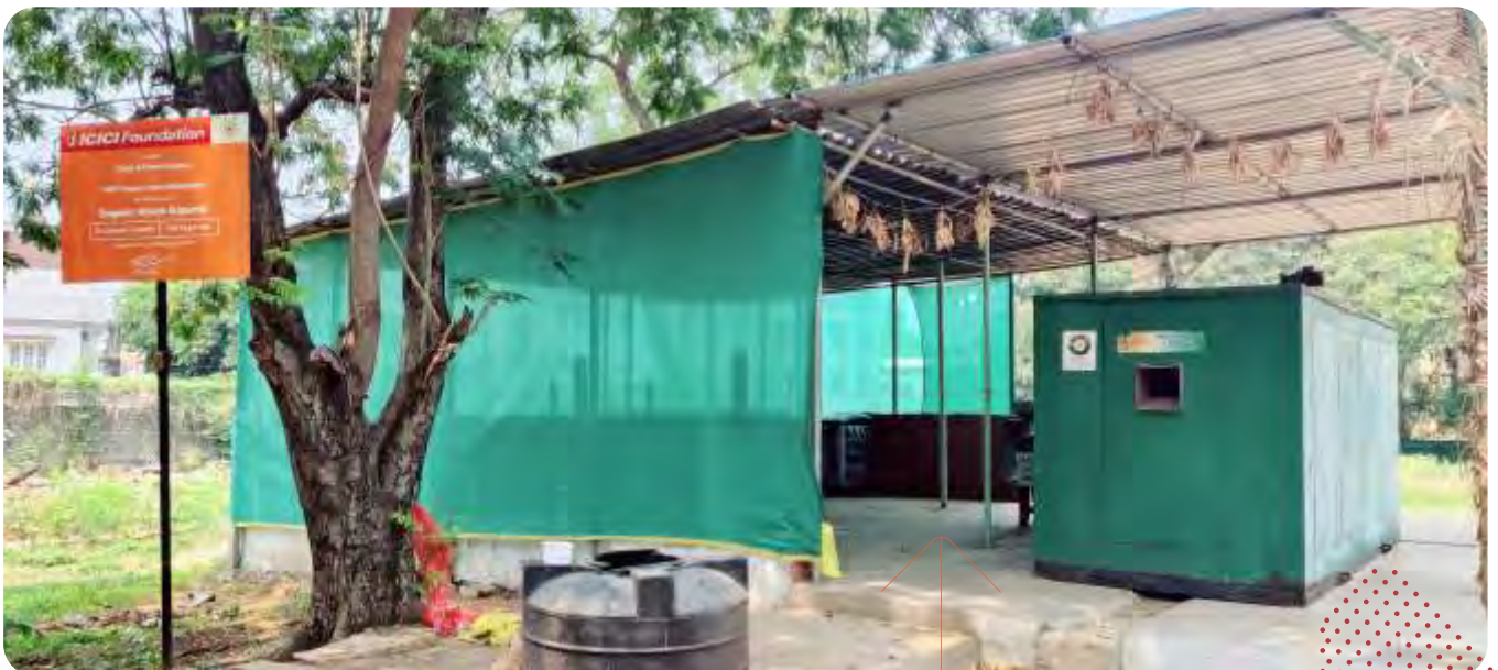
Bio-Digester at CRPF Group Centre, Hyderabad
