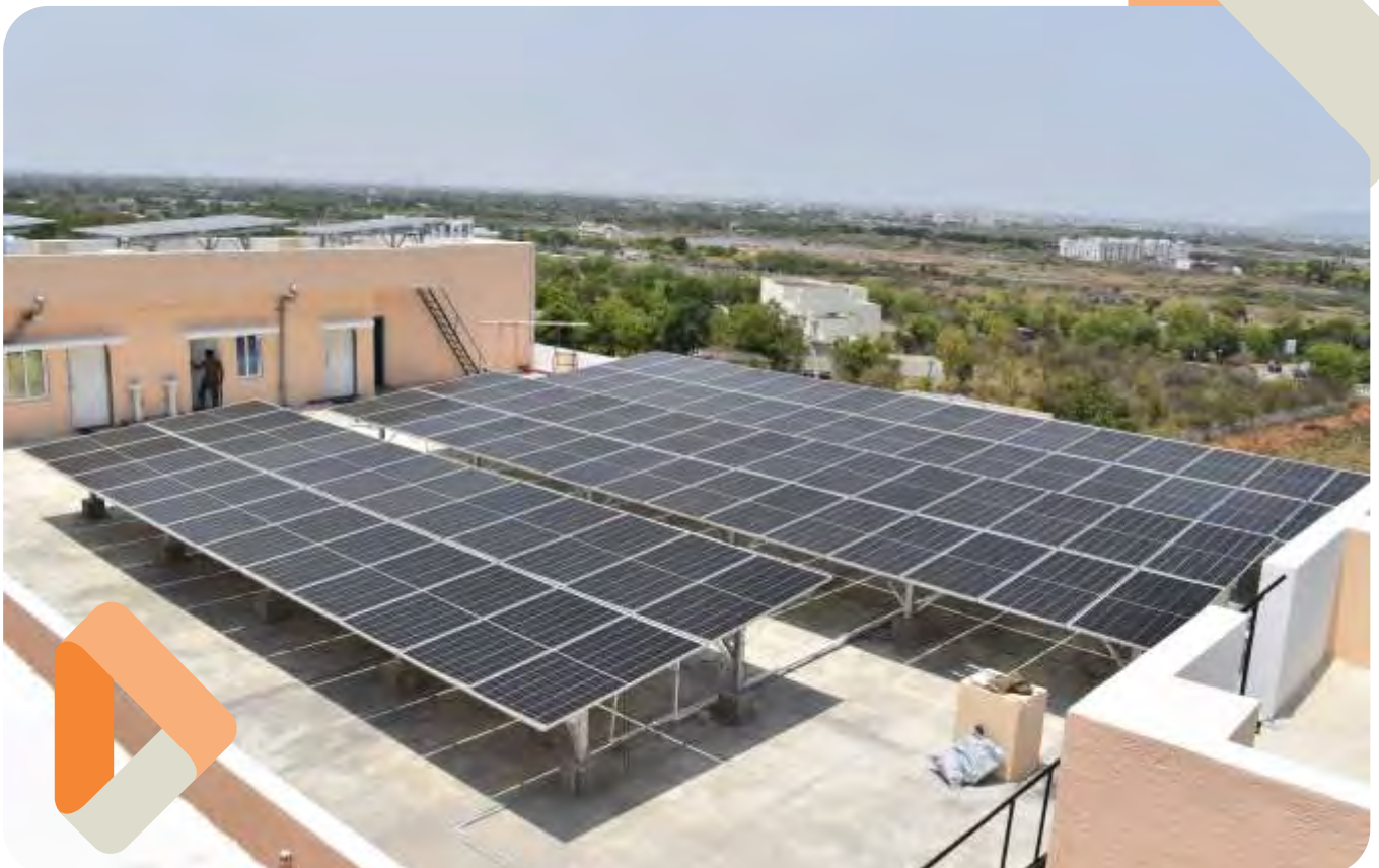
Solar Panel Support at PVRI, Kadapa
